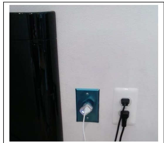
12VDC receptacle with triple USB ports ranging from 1-2.4Amps; 120VAC 20A rated dual receptacle; left: a wall-mounted 120VAC plug-in style eheat/envi unit
