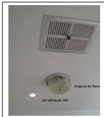
Bathroom DC-AC side-by-side lighting
